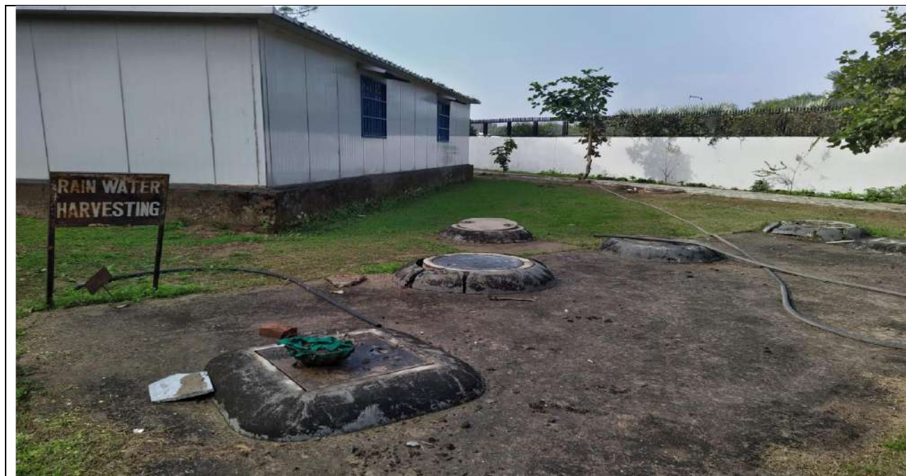
Fig. 5: Overview of Rain Water Harvesting System in College Campus
