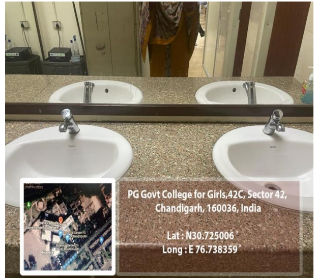
Push Puller Cock Taps in restrooms
