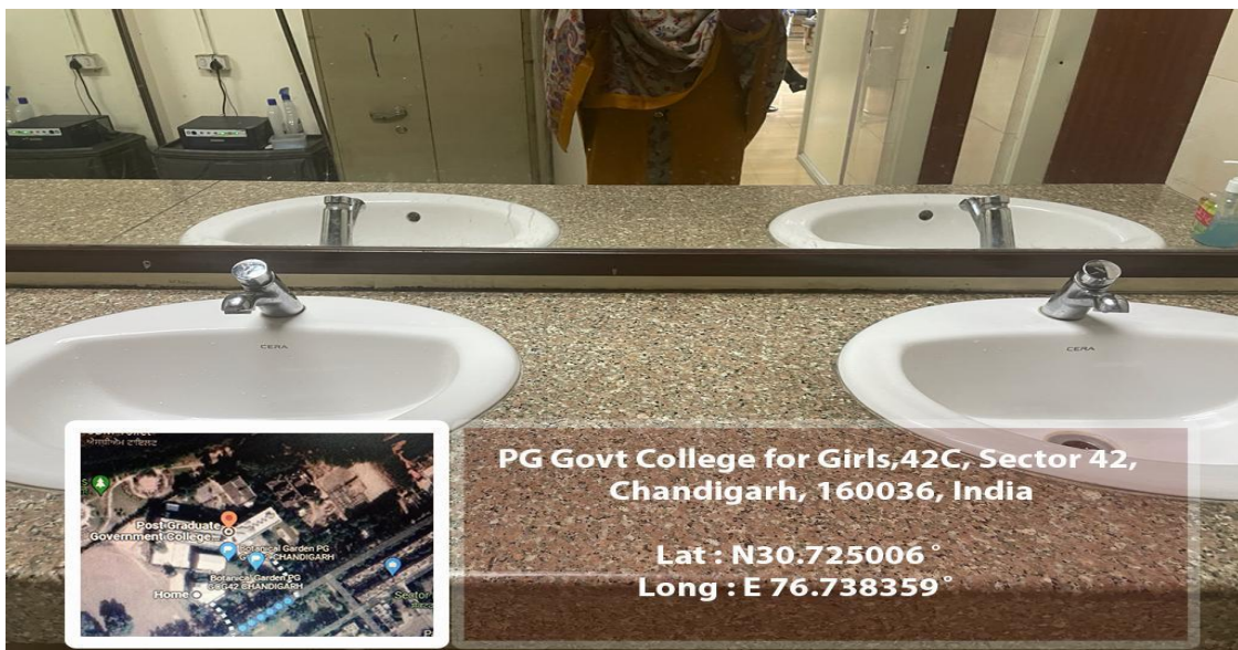
Push and Puller taps in washrooms
